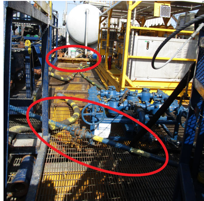
Egress routes not clear and free of obstructions
